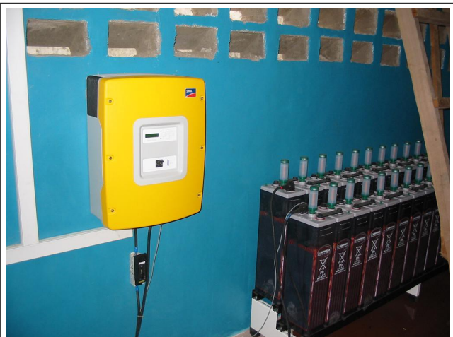
Sunny island and batteries
