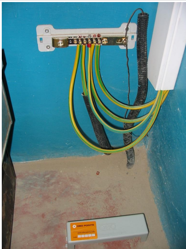
Common grounding point
